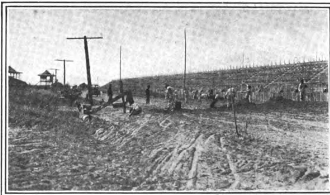
7—The surface of the course is being repaved throughout the whole circuit
